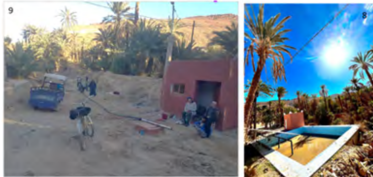
Figure 7/8. New Wells at Taghijit Oasis, Ain El Ansar with Solar Energy at Ifrane Source: Mohamed LOUAZANI, 2023
